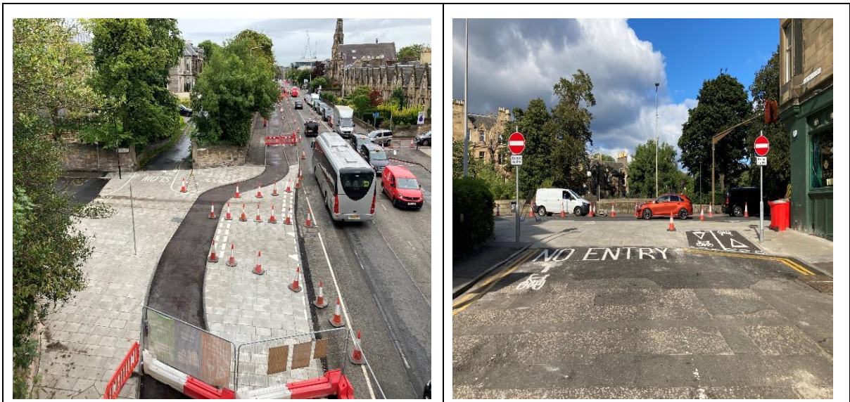
Section 1 - New junctions with continuous footways at West Coates and Roseburn Gardens
