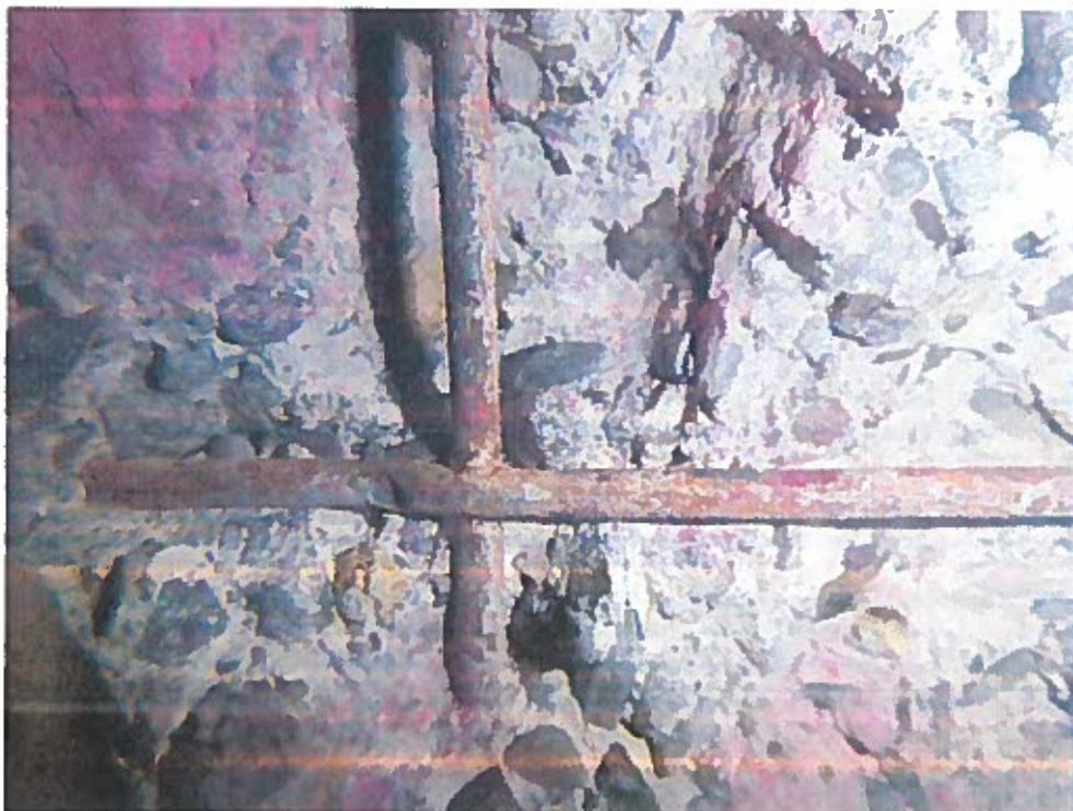
Plate 13. Area 1, Soffit of Slab Concrete Cover Removed to Expose Reinforcement
