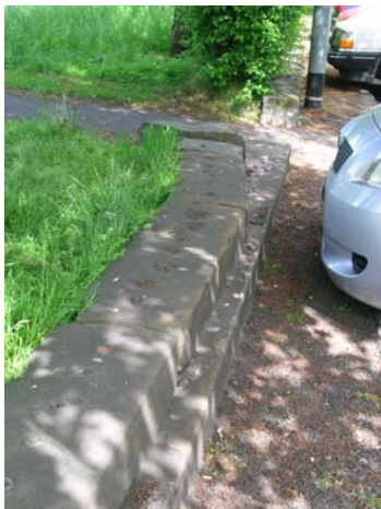
Shifted cope stones, Atholl Crescent
