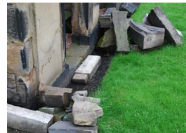
One of many groups of broken stonework
