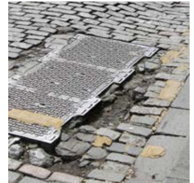
Damaged road surface
