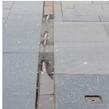
Damaged paving and shoddy repairs
