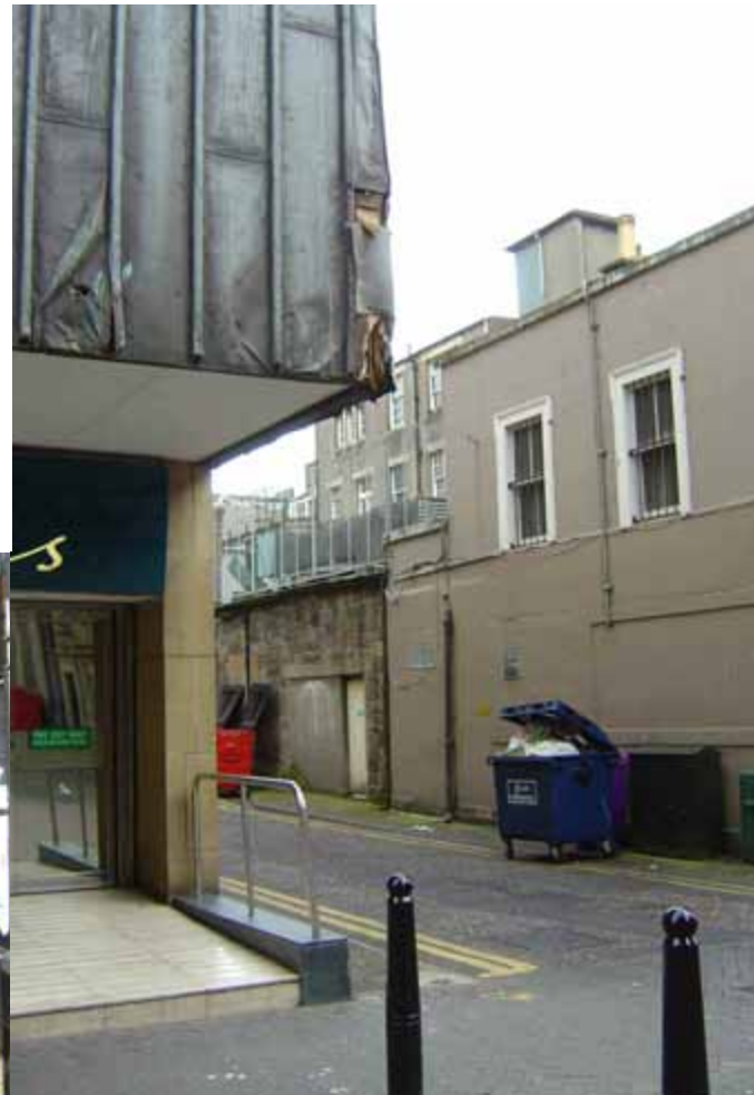
property damage due to poor servicing
