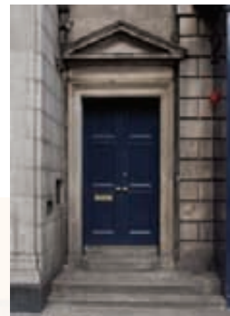
140 Princes Street. Detail of remaining fragment of rusticated stone (right hand side of doorway)
