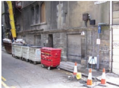
Early single storey masonry wall incorporated into the rear of the Old Waverley Hotel, August 2007.
