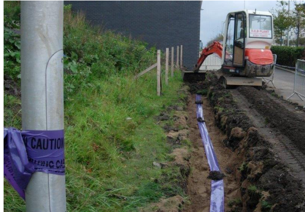
Smaller duct protecting the cable between the main duct and the lighting column.
