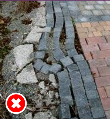
Pavement failure due to insufficient edge structure
