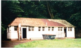
June 1999 Vandalised and neglected
