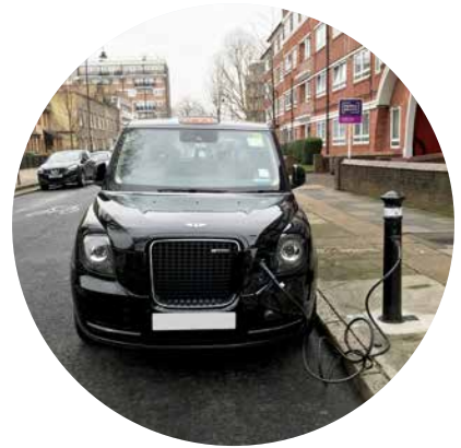
Electric vehicle charging points
