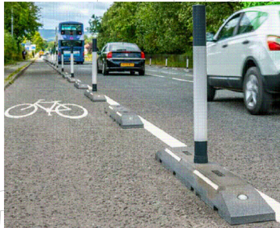
FIG 1. ROSEHILL NARROW CYCLE LANE DEFENDER UNITS - TO PROVIDE TRAFFIC SEGREGATION. PRODUCT 2.0M IN LENGTH & ARE BOLTED INTO CARRIAGEWAY WITH 5M GAP. NOTE CONTINUOUS WHITE LINING ON ROAD SIDE OF DEFENDER.
