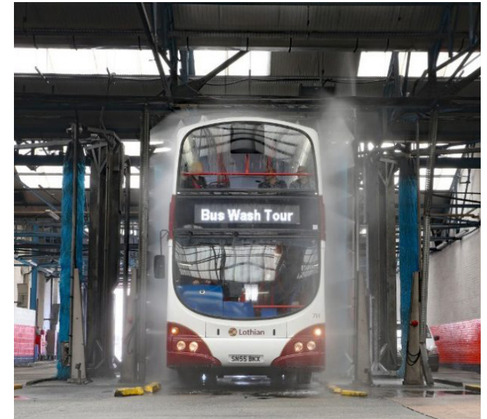
Figure 50. Bus Wash water recycling system | Lothian Buses
