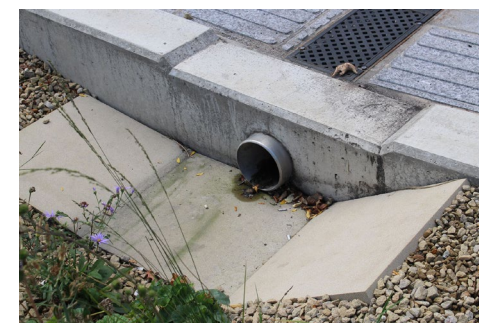
water inlet via a piped connection
