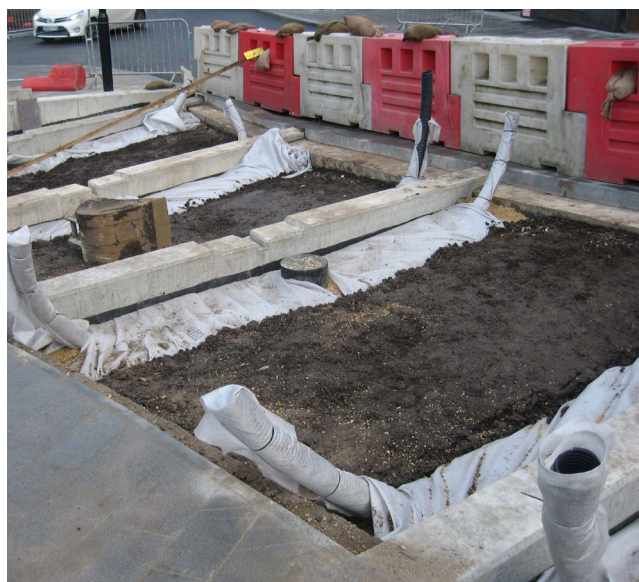
Figure 14. Engineered soil used in rain gardens for Sheffield Grey to Green Scheme | Sheffield City Council
