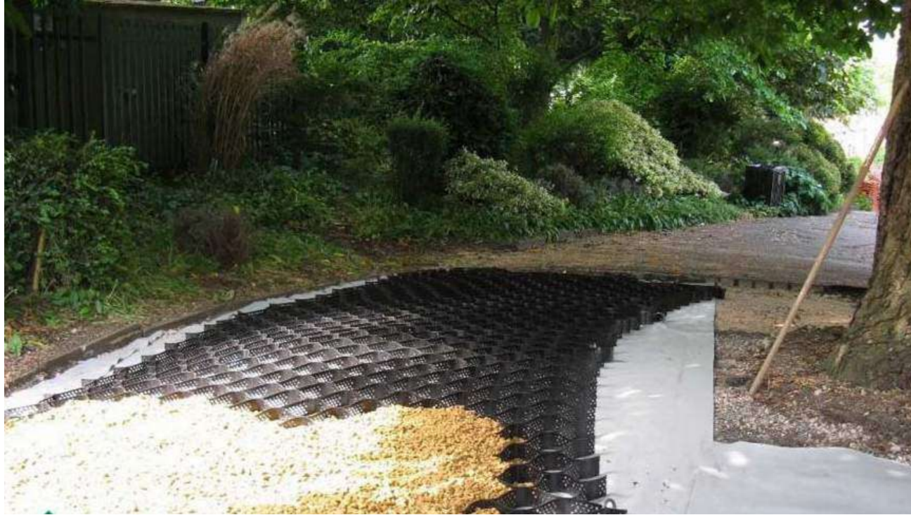
Self-binding gravel paths built upon a root protection mesh with help protect the roots of existing trees from damage arising from soil compaction and help define a hierarchy of paths within the park
