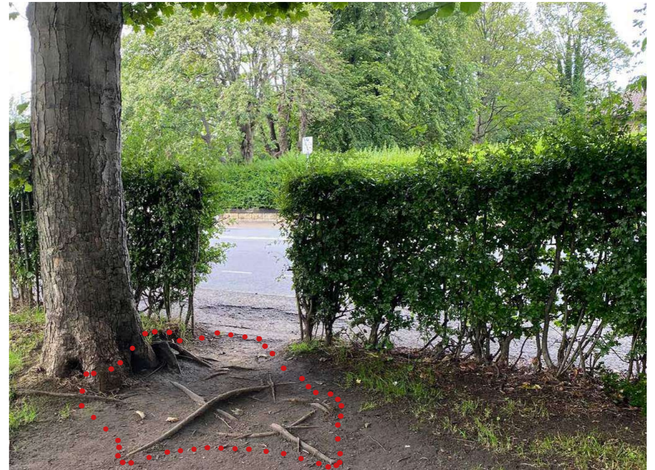
An informal entrance into the park along its eastern perimeter - with damage to tree roots highlighted
