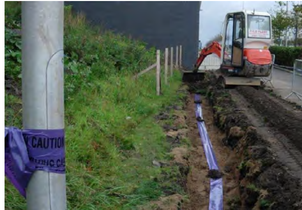
Smaller duct protecting the cable between the main duct and the lighting column.
