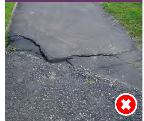
Failed Asphalt Paving
