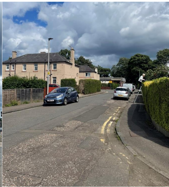
Example of worn markings at Featherhall Road and Featherhall Terrace
