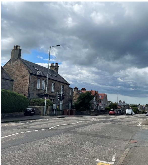
Example of worn markings at Saughton Road North
