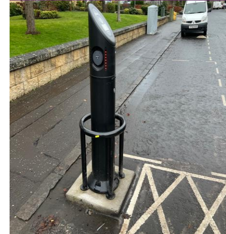
Figure F8.8 – Barriers to protect the chargepoint must not impede wheelchair access
