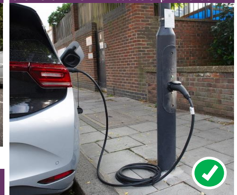
Figure F8.22 - Charging socket parallel to the kerb. This will reduce trip hazards
