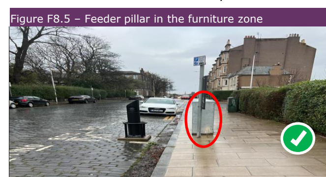
Figure F8.5 - Feeder pillar in the furniture zone City of Edinburgh Council
