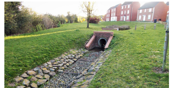
Figure 14. Armoured section of swale, Leicester | Susdain
