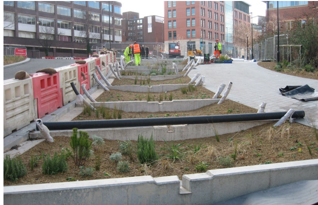
Figure 11. Swale constructed on a slope | Sheffield City Council
