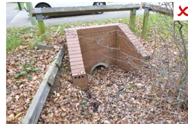
Figure 39. Blocked headwall outlet | Abertay University
