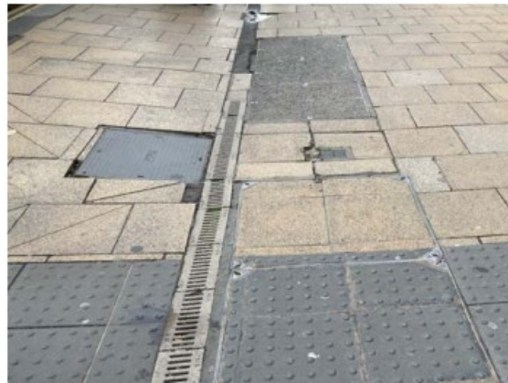
Low quality, easily damaged pavement surfaces
