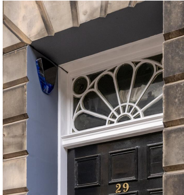
Security alarm box from primary elevation
