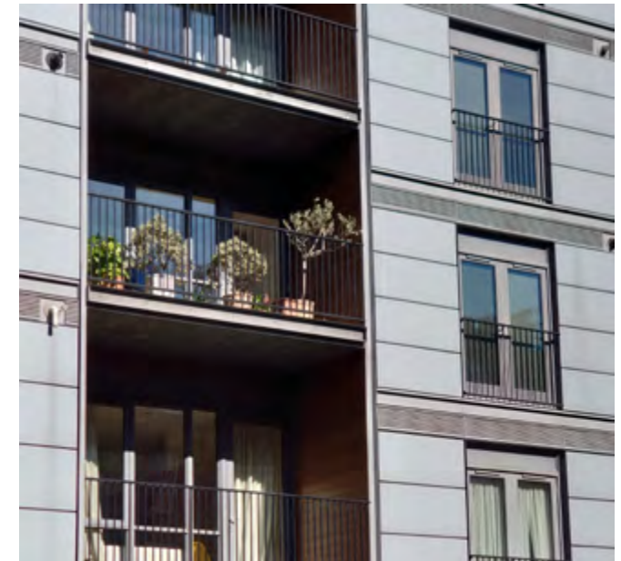
High quality detailing: metal cladding - Carefully detailed metal cladding on the rear wall of new flats in the New Town creates a variety of textures and a rich relationship of solid to void.
